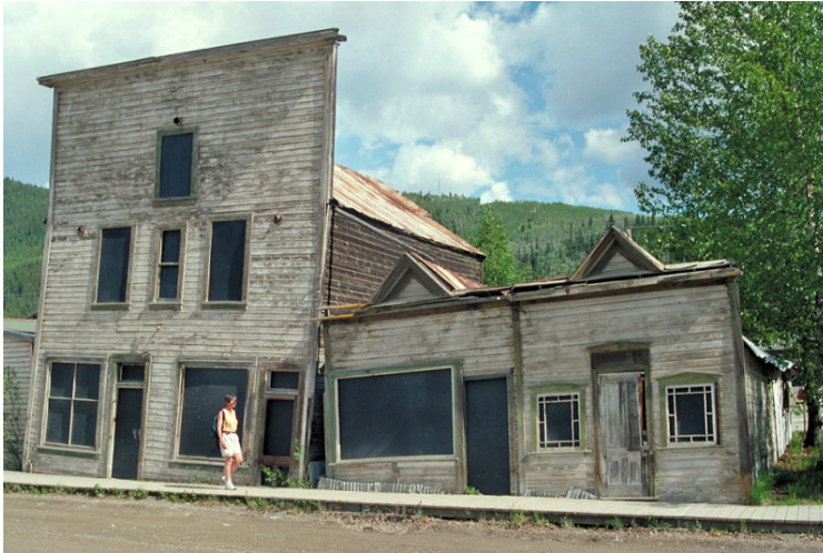
Permafrost damage, Alaska
