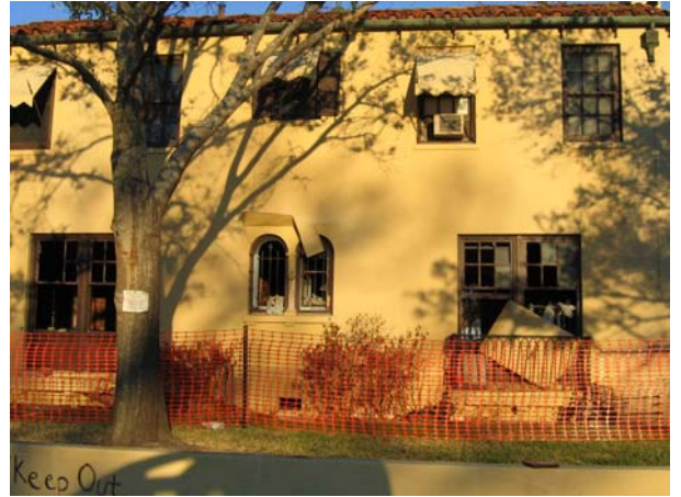
Damaged structure too large to relocate
