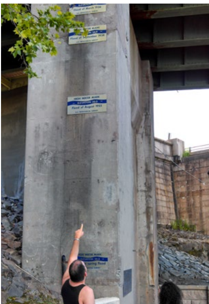
Multiple flood levels of the Connecticut River are shown in downtown Hartford.
