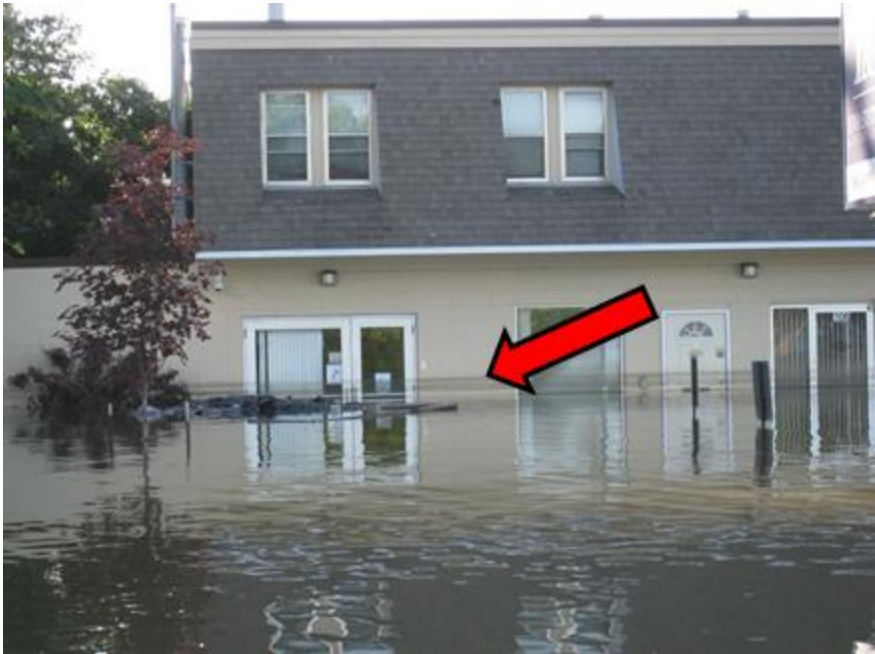
Figure 6- HWM from silt on a building during June 2008 flooding. Coralville, Iowa
