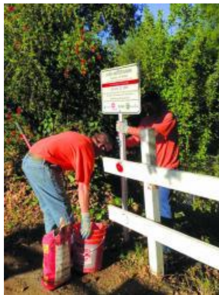
Figure 4- A high water mark being installed. Courtesy of Brian Jacobson, City of Roseville, CA
