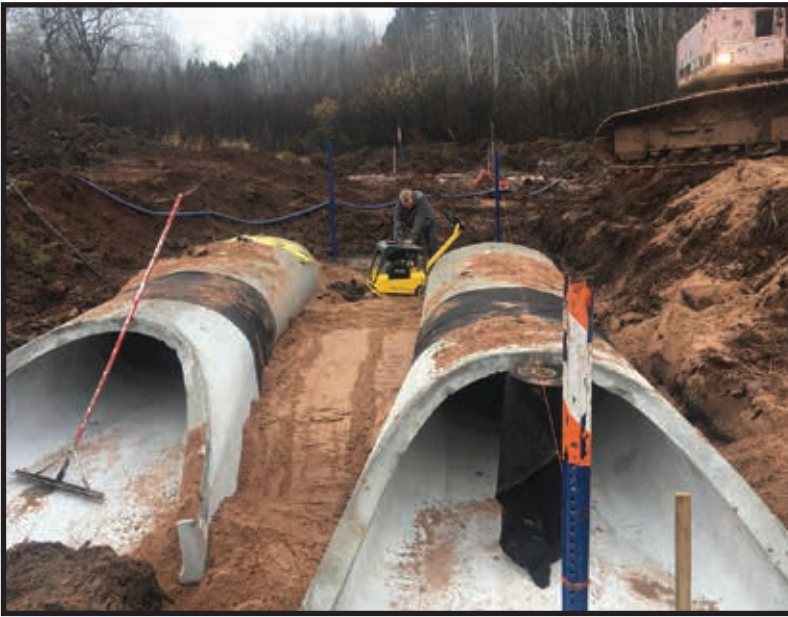
Bad River staff replacing a culvert on a tributary to Sucker Creek, which was regularly overtopped by water during spring floods. Funds were obtained through an EPA Great Lakes Restoration Initiative (GLRI) grant. (Photo by Eric Andrews, Bad River.)
