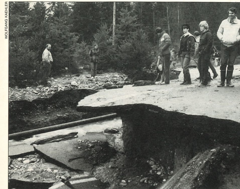
Property losses from floods are not limited to buildings. The ground under this road in Hollywood Hill, Washington, was washed away by torrential rains.
