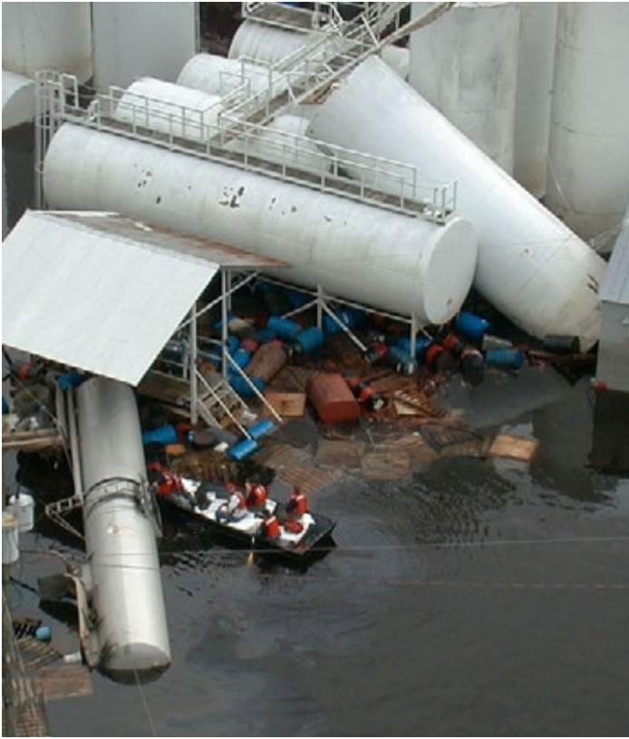
A hazmat team checks damage and oil contamination from flooded propane tanks. - Franklin, VA, 1999, Liz Roll/FEMA.
