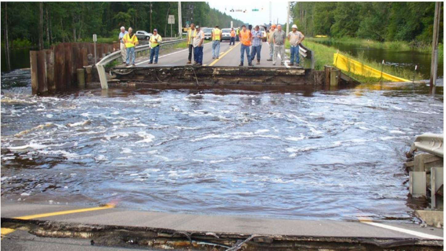
A flood on the St. Mary's River severed an arterial highway, US 301. - Nassau County, FL, 2012, Keith Gaston.
