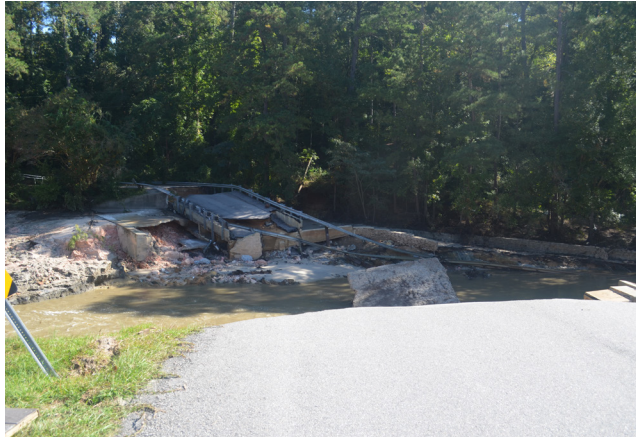
Figure 5.2. Cary Lake dam failure (when this dam breached, 15 properties lost roadway access to the properties) (Maria Cox Lamm)
