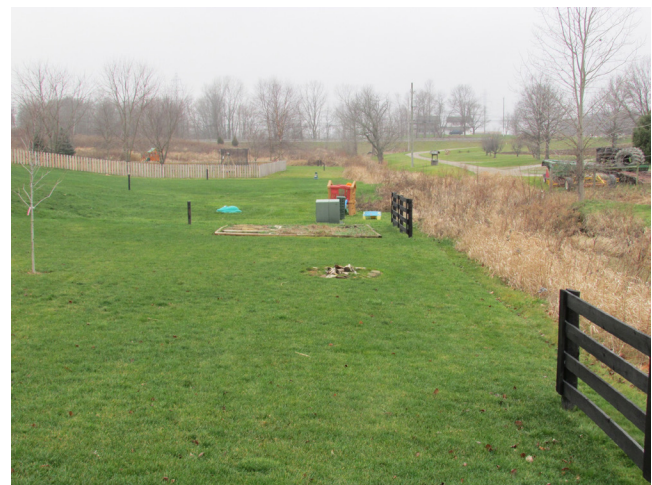
Figure 5.5. Non-elevated, pad-mounted transformer in the floodplain very close to the flooding source (Chad Berginnis)
