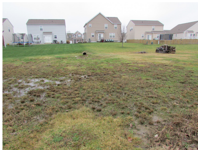
Figure 5.6. Wood debris stored in a stormwater retention area could clog the drainage outlet, threatening the integrity of the retention area berm and causing more significant flooding (Chad Berginnis)
