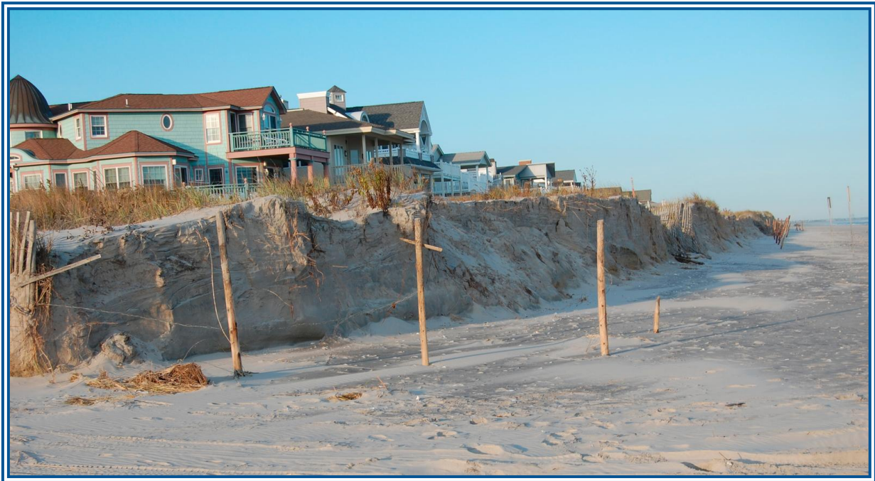
Damaged dunes from Tropical Depression Ida show that both dune volume and height are keys to determining the level of protection a dune provides (photo from FEMA library, Elissa Jun/FEMA.)
