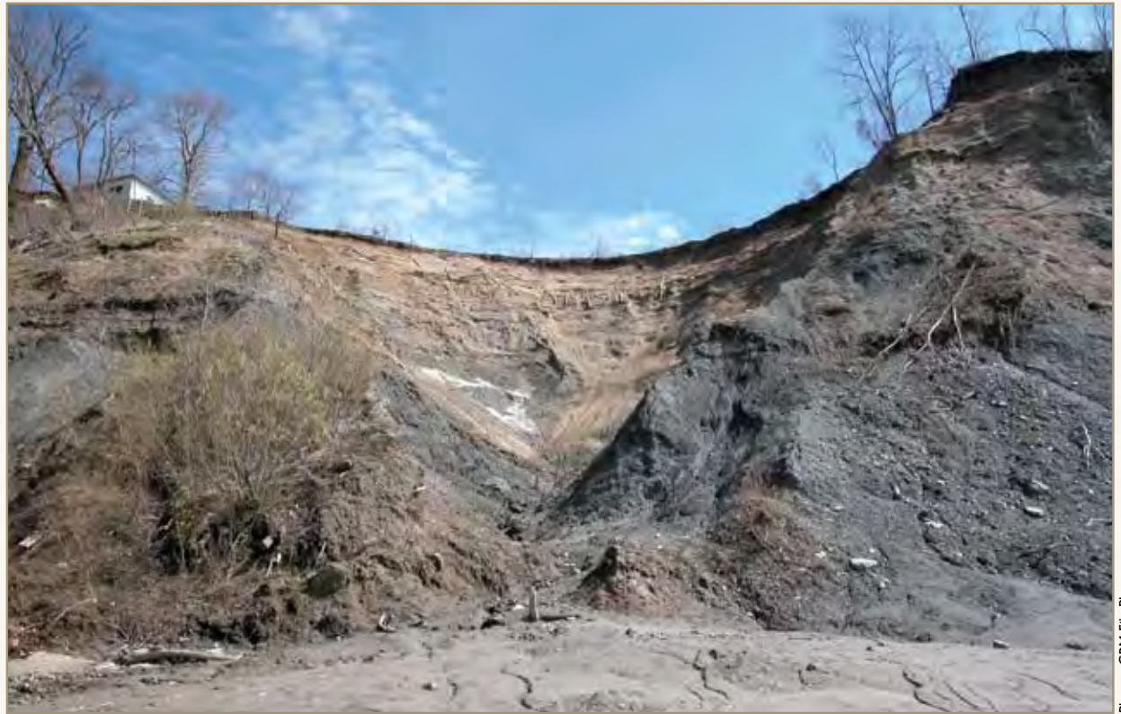
In this area in North East Township the sandy layer is especially deep, making it more susceptible to collapse.
