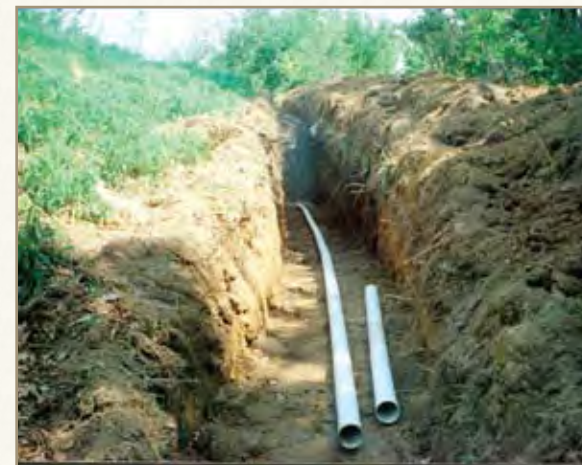
This is part of a drainage system designed to intercept surface runoff and groundwater. A drain (not shown) was installed in the low part of the yard.
