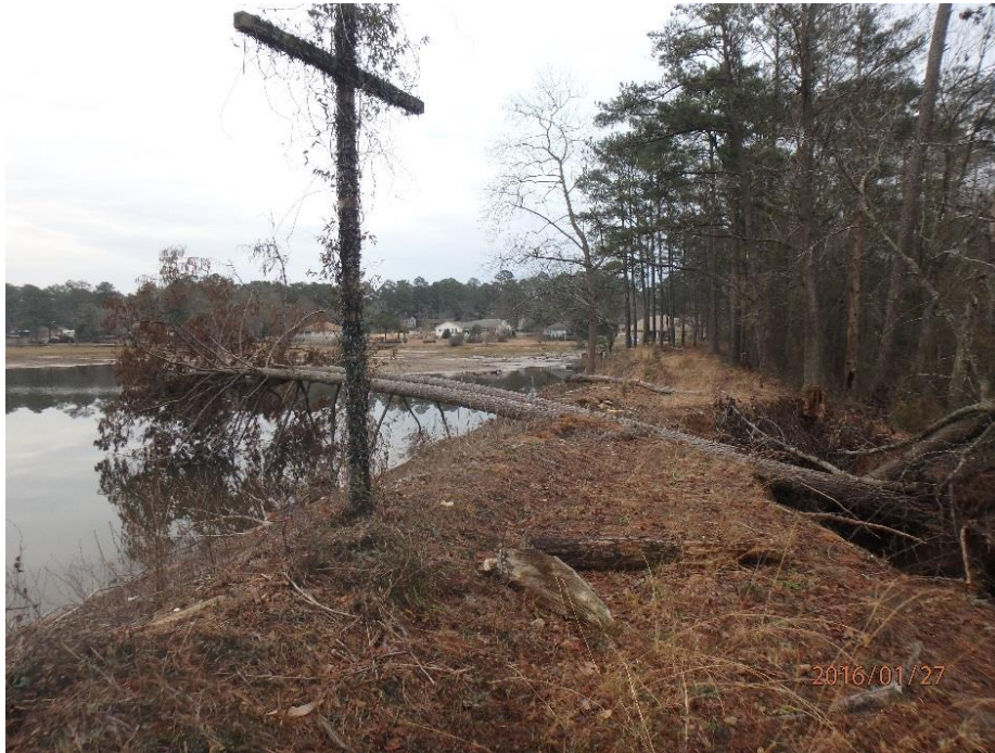
Figure 13. Overtopping Failure Exacerbated by Heavy Vegetation at Sunview Lake (Source: FEMA 2016)
